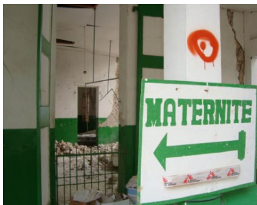
Maternity Ward at Jacmel Hospital reduced to rubble
